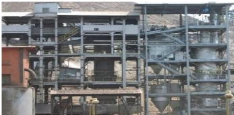
Fig. 2 Shaft furnaces at SMZ, a.s. Jelšava
